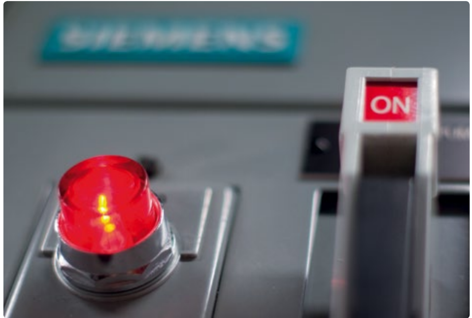
If an incident occurs an immediate and effective respond is needed
