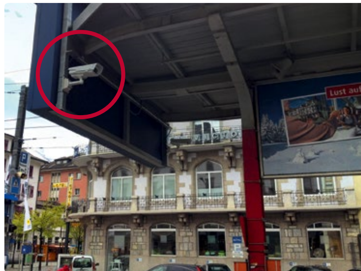
An Axis P 1344 E in use at Brig station
