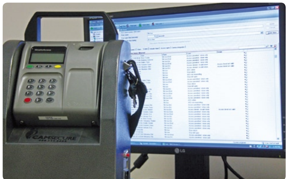
Data from the fingerprint reader is integrated into the security management software
