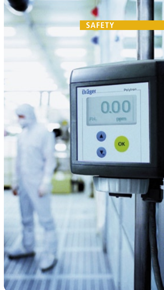
Stationary gas detection systems reduce the risk of hazardous incidents.
