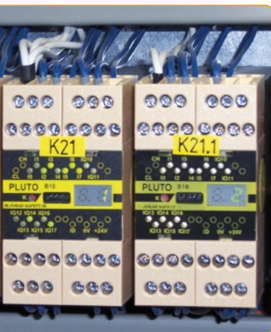
Fig. 2: The Pluto B46-6 and Pluto B16 safety PLC's with connected BT51 expansion relays are accommodated in the control cabinet and supervise the safety of all equipment. ▼
