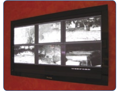
The thermal images can be shown on any of the screens inside the house.
