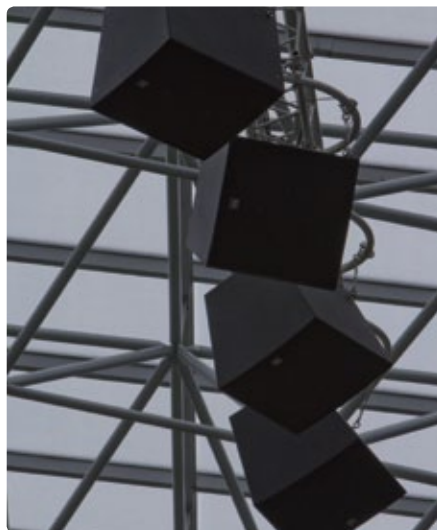
At NSK Olimpiyskiy Stadium, EV-Innovation Series Speakers, EV CPS Power Amplifiers and EV N8000 Digital Matrix build the backbone of the sound system.
