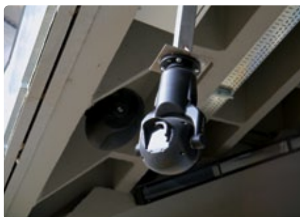
Vandal-resistant MIC 400 stainless steel cameras were installed close to the supporters
