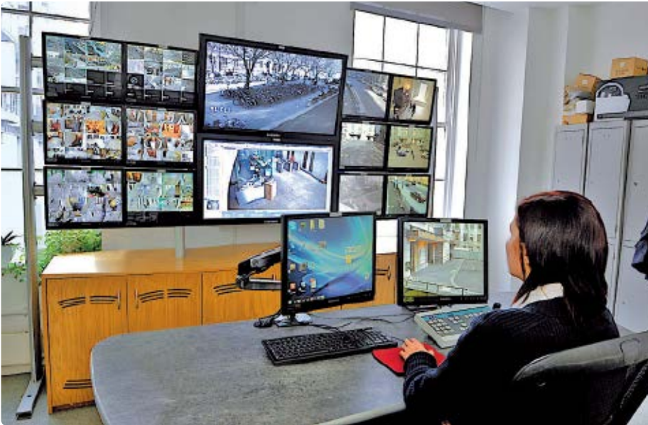
The images are available for the University of London Building Management teams and Balfour Beatty WorkPlace security team
