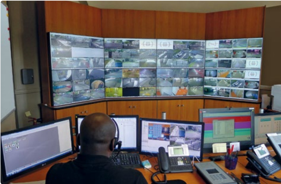
Several alarms can be shown simultaneously on the monitor wall
