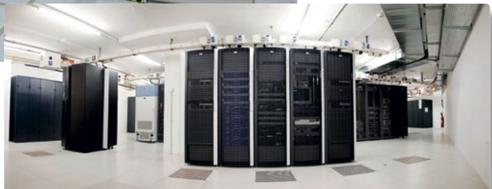
Aspirating smoke detection (ASD) from Siemens will provide the earliest possible warning even when the smoke is barely discernible to people ▼
