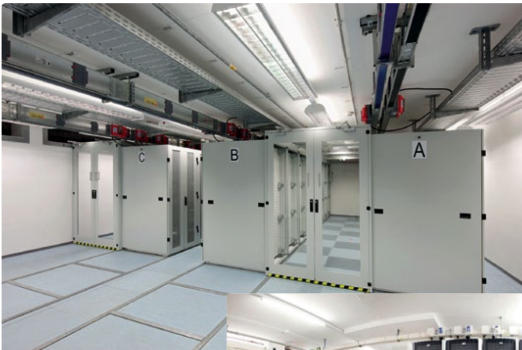
◀ Effective fire safety systems are a fundamental requirement in achieving maximum system uptime and availability
