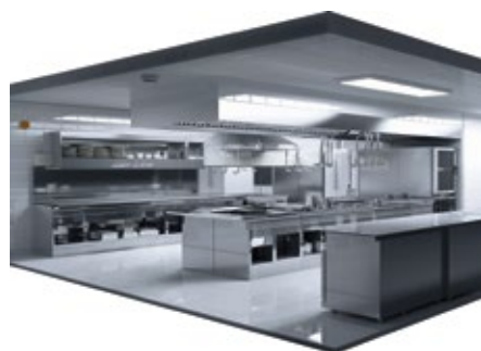
Due to the high fire load of open flames or frying pans, commercial kitchens are one of the most dangerous places in a hotel
