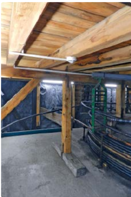
IQ8Quad detector in the bollard room
