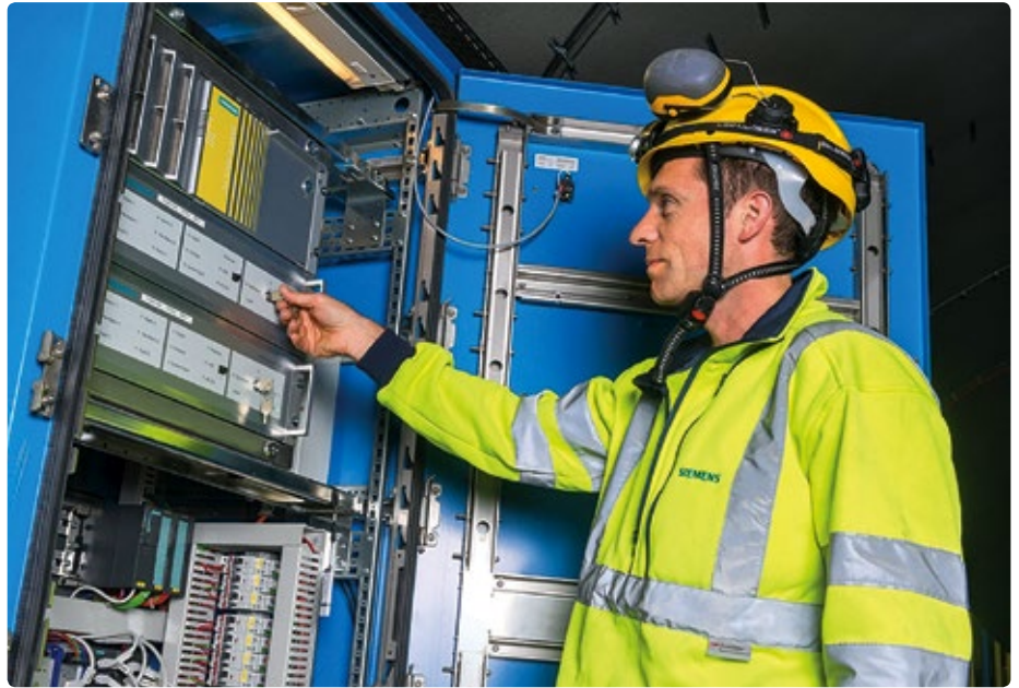
Marco Pradera specializes in tunnel fire safety for Siemens Building Technologies division
