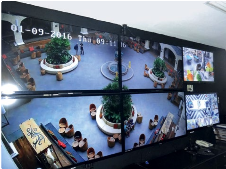
Thanks to the video surveillance system, the security staff can monitor the whole hotel
