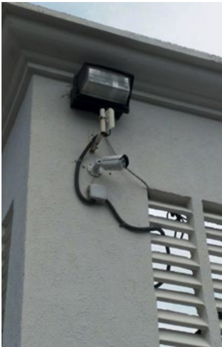
The installation process of the new security system was developed in phases. In the first stage, 89 Hikvision cameras were mounted. Later, 30 additional units were installed
