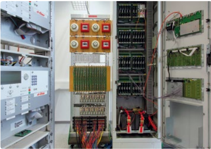
The MegaFoot lab is used to test the behavior of large, networked installations of up to 64 fire control panels
