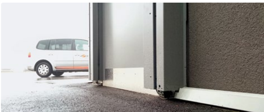
A TIM3xx guide rail-mounted 2D laser scanner from Sick protects the area under the cab
