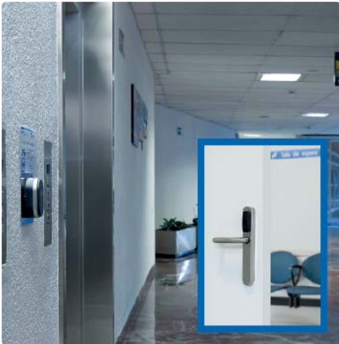
Access restrictions for lifts, doors and car parks are managed by Assa Abloy's SMARTair system components
