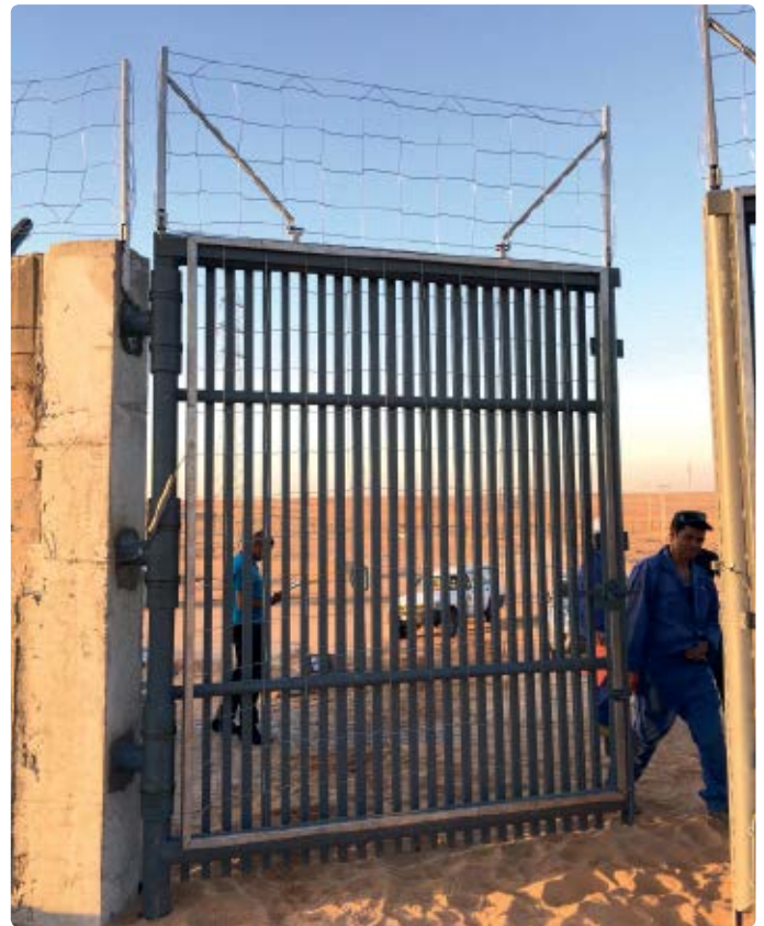
The Peristop sensor net detection system uses detection bent arm systems on the upper part to detect climbing
