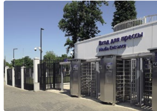
Bosch installed more than 2,000 cameras to safeguard the vast perimeter
