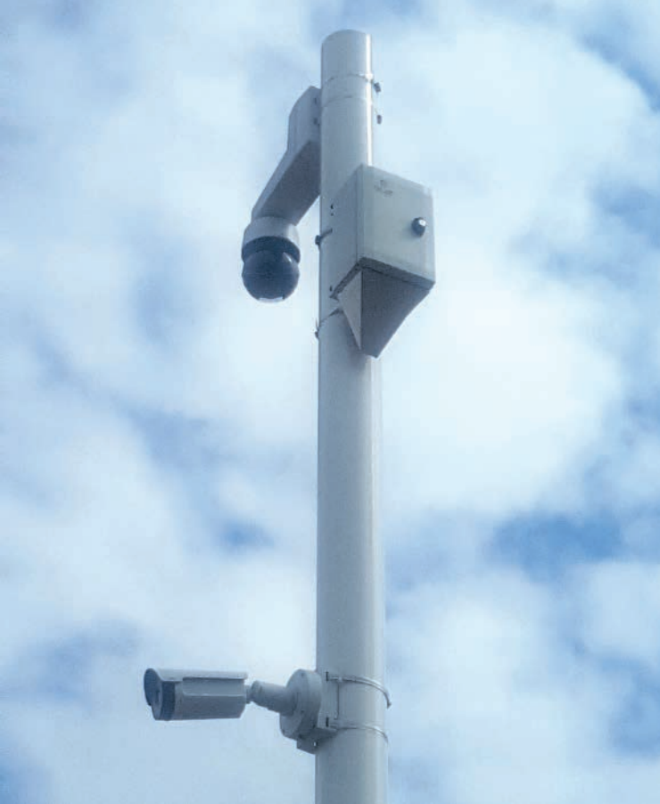
Danger recognition: A Slat Synaps 24V 3E IP with a built-in 60W high PoE injector and a fiber-optic media converter supplying and buffering moveable Axis dome infra-red cameras
