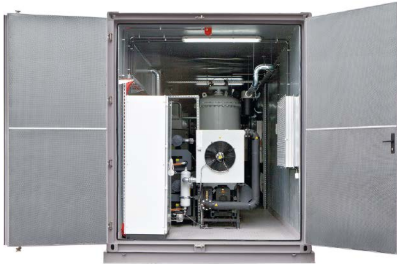
Almost the entire fire protection equipment is built into a compact container
