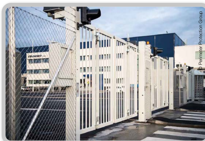
At Helsinki airport, Perimeter Protection Group installed EntraQuick quick folding gates and full-height turnstiles
