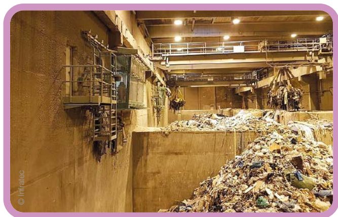
◀ Dresden based InfraTec provide the Waste-Scan and Fire-Scan systems that use thermographic measurement to detect hot spots
