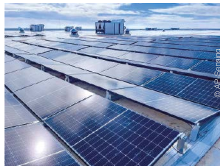
With a passive fiber optic cable used as a distributed temperature sensor, the system from AP sensing measures thousands of temperature points in real time, monitoring photovoltaic system temperatures
