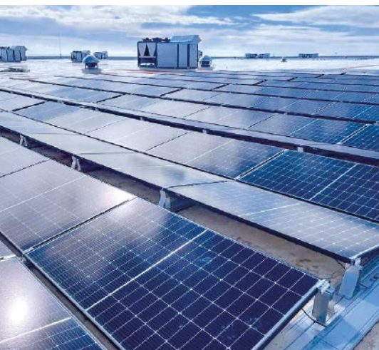
This project in Badajoz, Spain, highlights the effectiveness of AP Sensing's FO LHD system in PV panel monitoring
