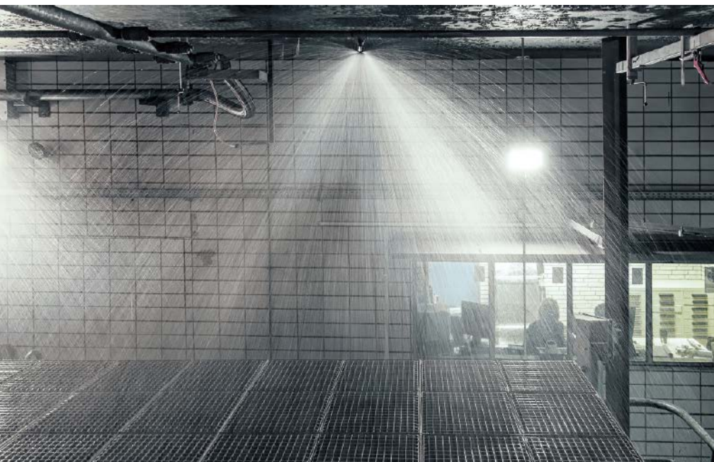
Good old-fashioned water sprinklers (here: thoroughly tested in the unique VdS laboratories in Germany) have been found to be very effective in preventing the spread of fire in lithium-ion battery storage areas
