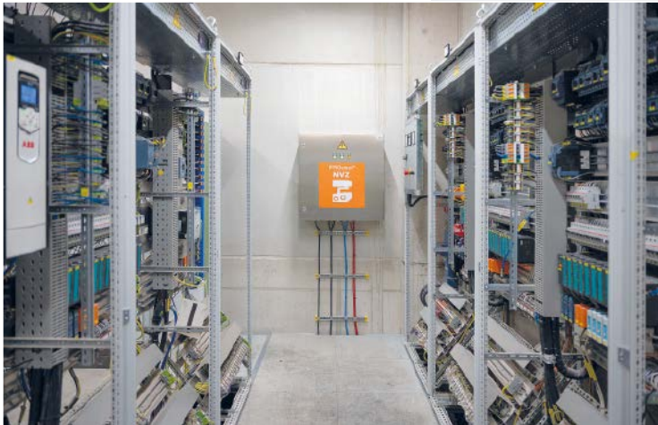
Orglmeister provides the entire system technology for safe monitoring, which is then housed in a small control cabinet in the building's electrical operations room
