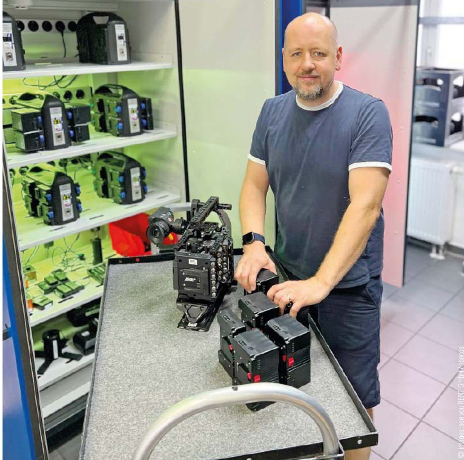
At See you rent, lithium-ion batteries are safely stored in Ion-Line cabinets from Asecos
