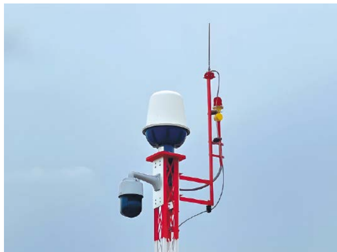
One of the newly installed HDR311 high definition radar units integrated with Navtech's AdvanceGuard software platform. The system delivers real time wide area monitoring, automatic rule based alerts, and seamless camera cuing for rapid airside incident verification.
