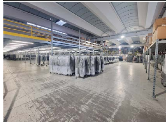
Addressable detection placed around the overhead trolley system uses automatic drift compensation to maintain reliable sensitivity despite constant air movement and fibre particles
